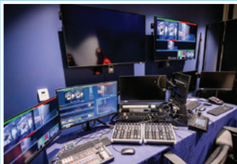
New control room.
